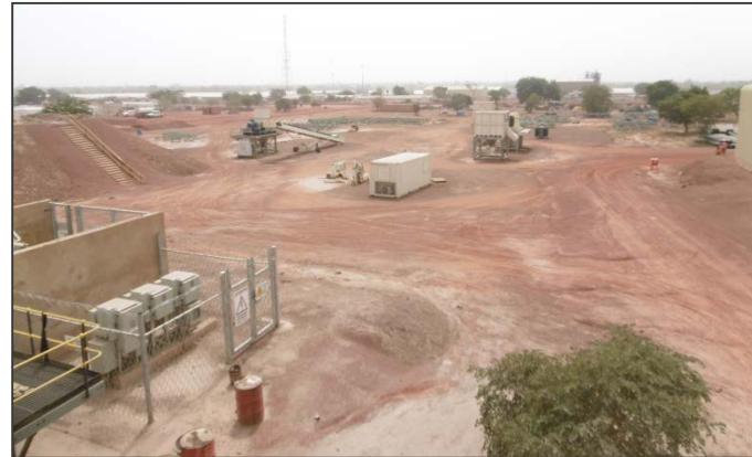
Feed Preparation Circuit - Before
