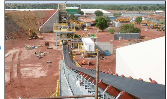
Feed Preparation Circuit - After
